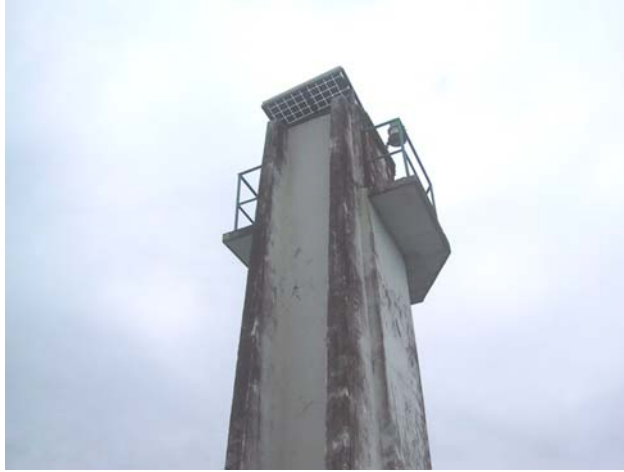
Figure 20. The navigation light tower and existing solar panel at the port entrance.
