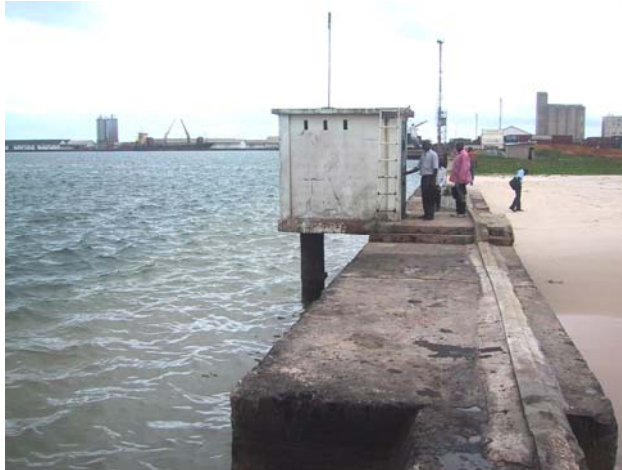
Figure 18. Old Tide Gauge Hut with sand build up on either side of jetty.
