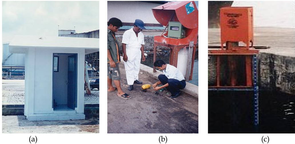
Figure 3. The existing tidal stations are still in different type of buildings. To meet high quality observations, efforts have been made to improve all station into the standard buildings as shown in (a).
