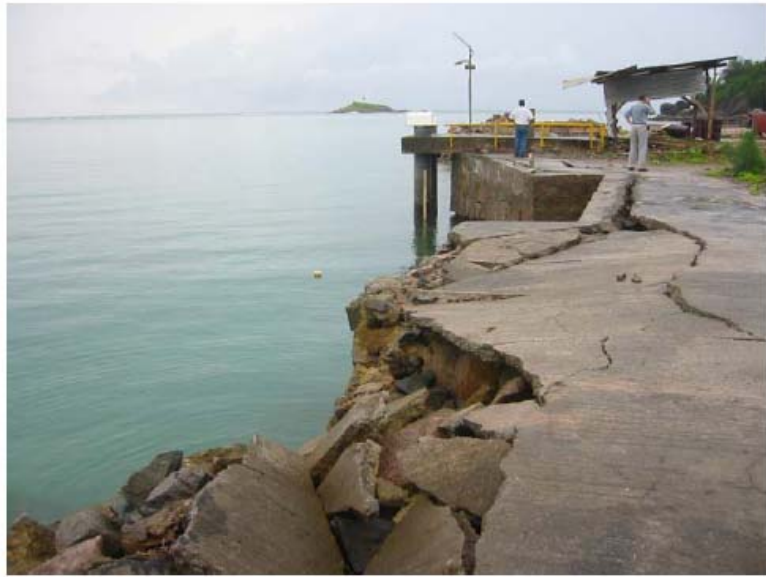
Fig 7: Structural Damage by the tsunami, 2005
