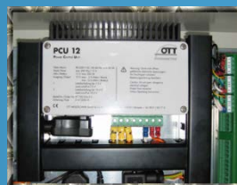
Power Control Unit
