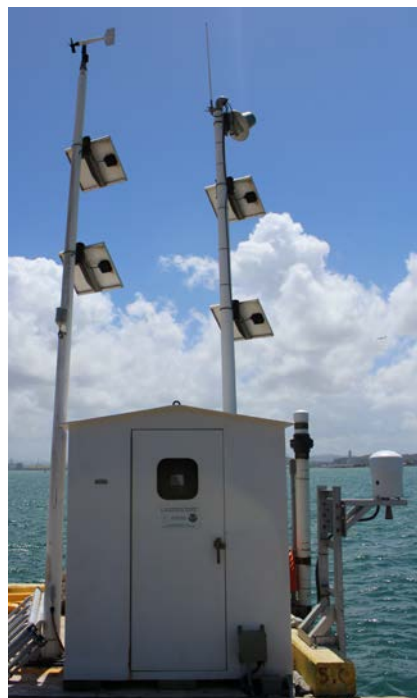
NOAA NWLON Station in San Juan, Puerto Rico with both acoustic (in back) and microwave sensors installed
